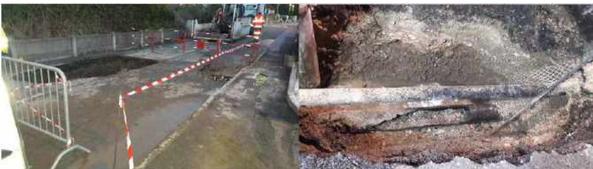
Rupture canalisation DN 200 mm Montanot
